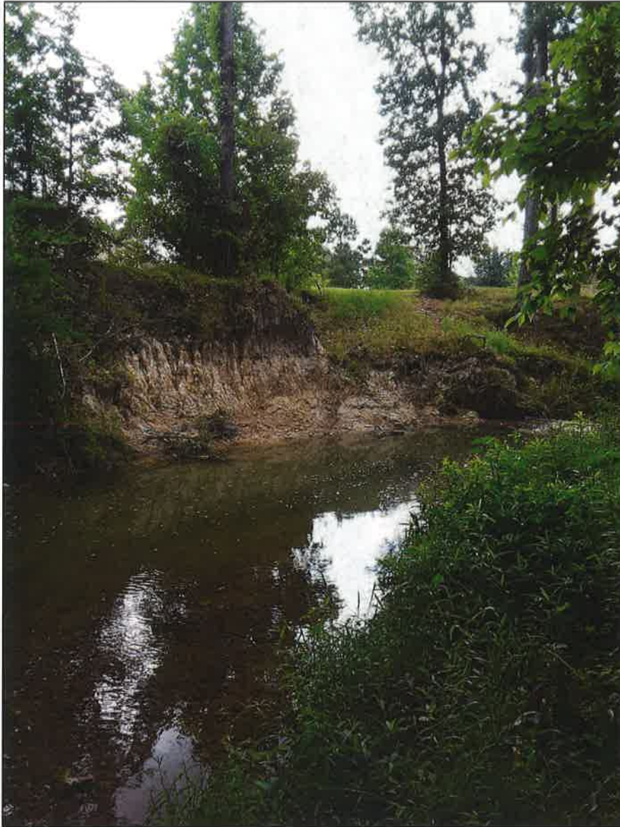
Photograph 2: View of Section B from south bank facing north bank showing severely eroded, vertical bank.
