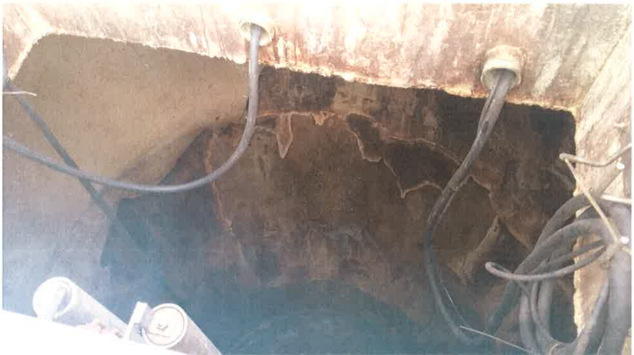
Lift Station No. 2 – Wet Well – Coating Failure
