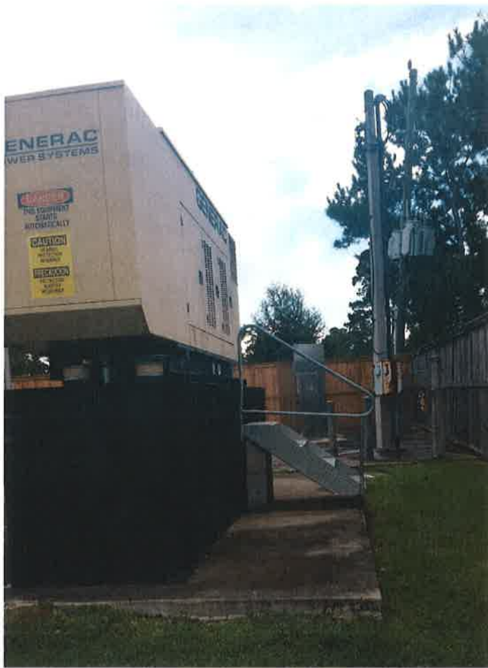
Lift Station No. 1 – Generator – Lack of Safe Maintenance Walkway
