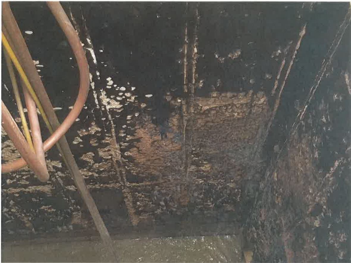
Lift Station No.1 - Wet Well – Coating Failure
