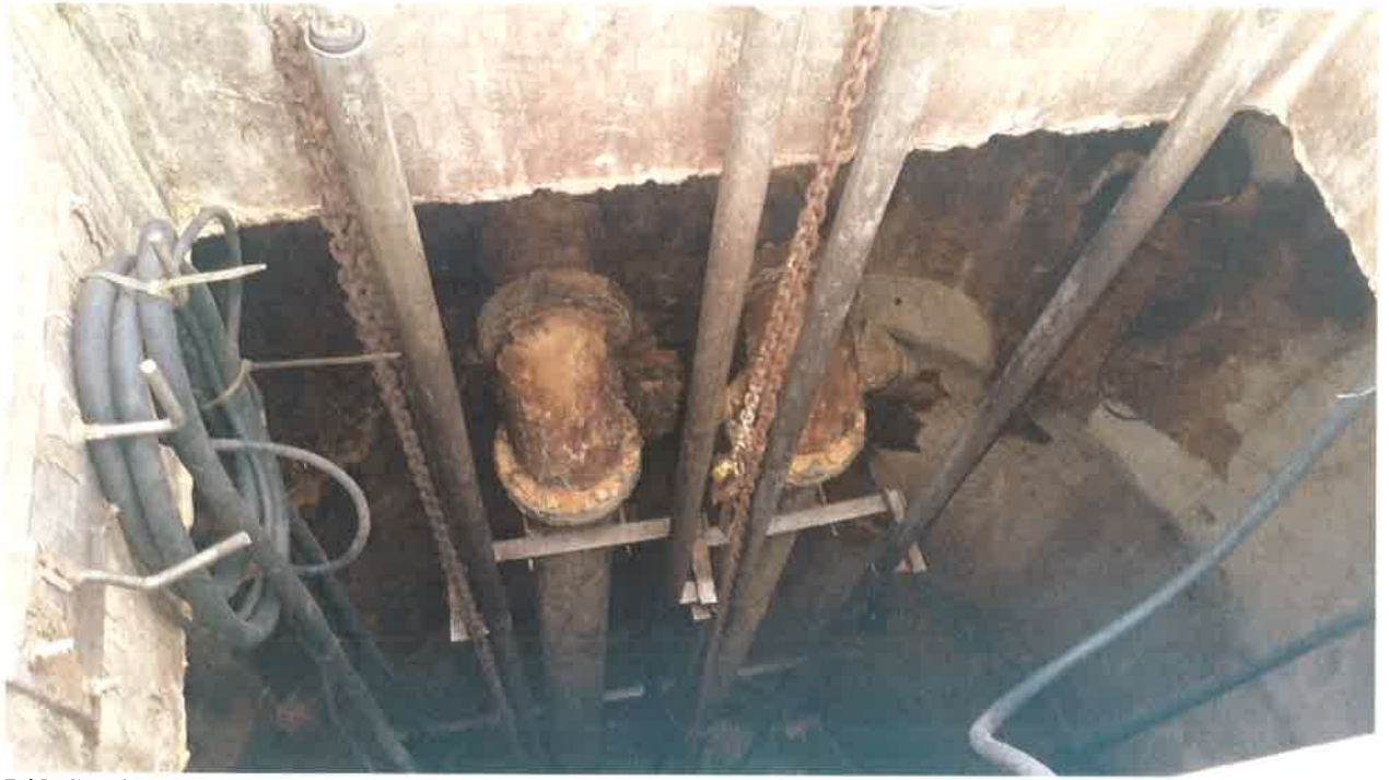
Lift Station No. 2 – Deteriorated Piping/Rails
