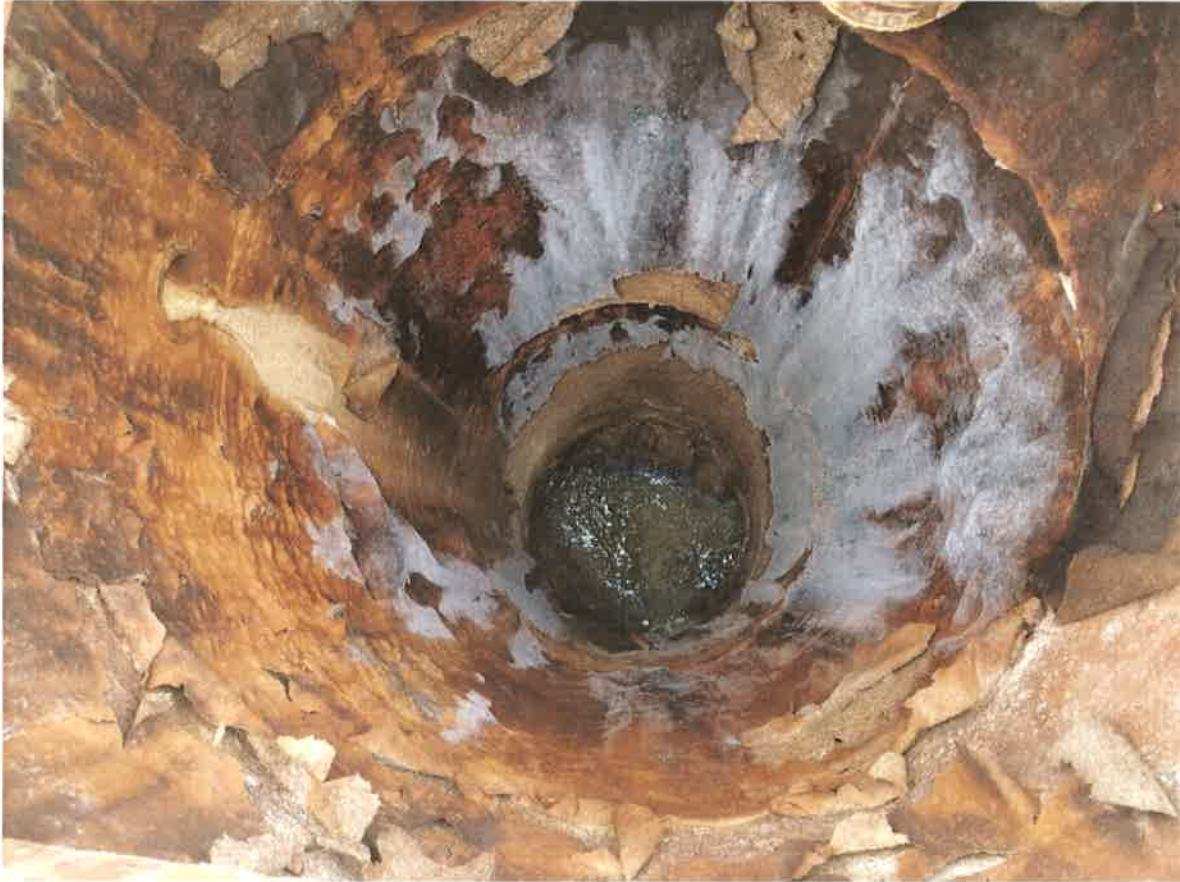
Lift Station No. 1 – Adjacent Manhole – Coating Failure
